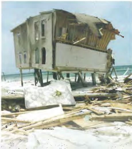
Damage to beachfront home from Hurricane Dennis.
